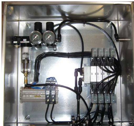
Example of an air cabinet
